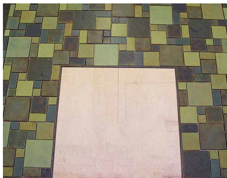
The new facing uses handmade Syzygy tiles; Michelle laid the pattern out on the floor first to finesse the color distribution and grout lines.
